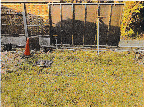
Photo no. 2 Along the lots boundary consisted with metal fence wall, which sealed up at the bottom.
